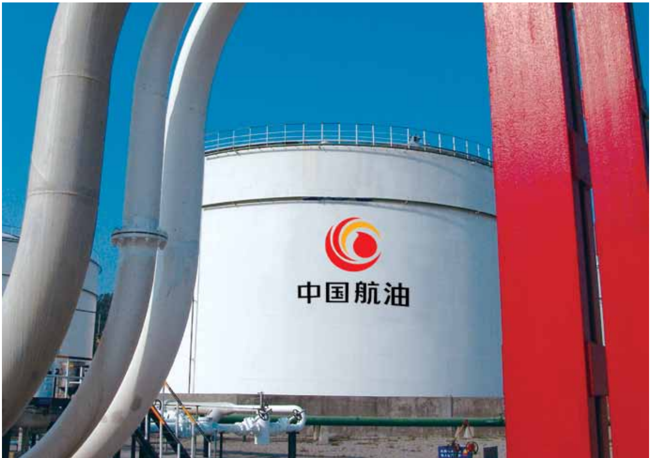
Oil storage facilities at CNAF CNAF 储罐设施
