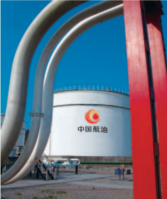
Oil storage facilities at CNAF CNAF 储罐设施
