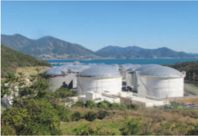
OKYC tank farm in Yeosu, Korea OKYC在韩国丽水的储罐
