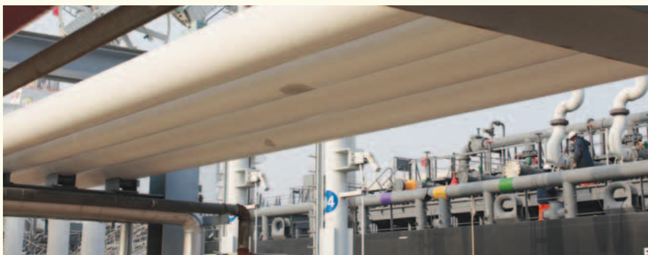
Pipelines at Shanghai Pudong's discharge port 浦东机场卸油码头输油管线
